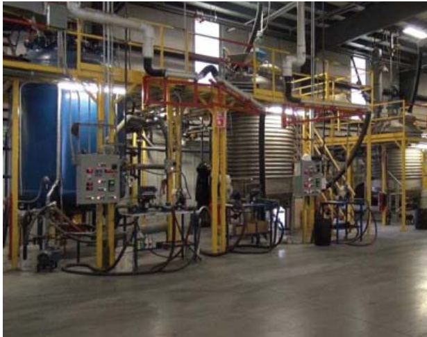
Reactors at JACAM facility
