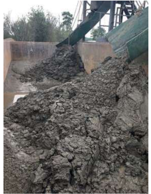
Optimized solids control equipment in combination with EnerSEAL HDD properties resulted in dramatic waste reduction (above)
