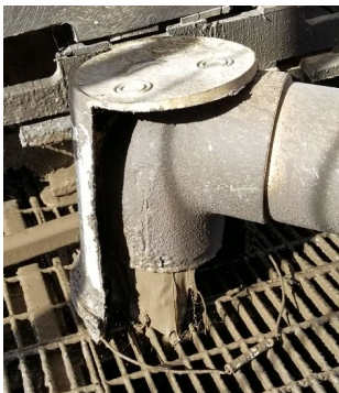
Figure 5: Centrifugal pump discharge
